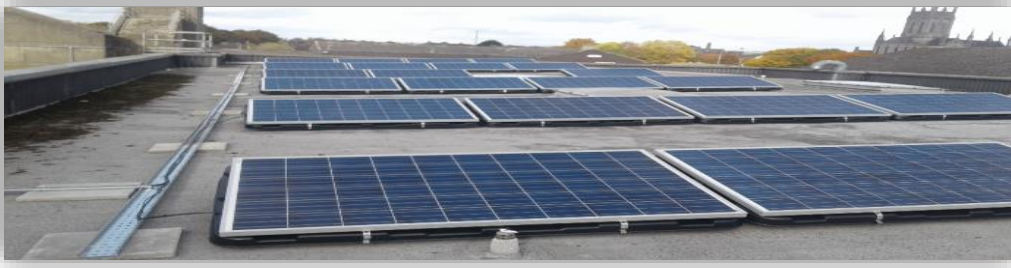
Kilkenny Fire Station 6kWp solar photovoltaic panels
